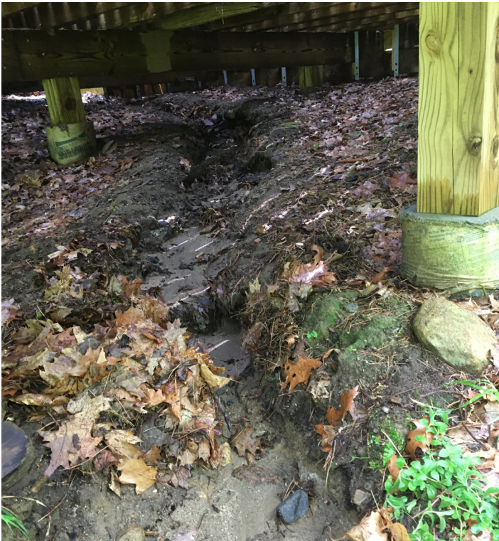
Figure 3: An example of erosion in Arrowsic (photo credit: Jack Witham)
